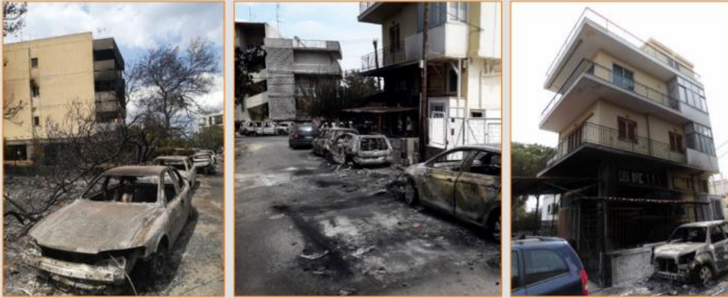
Destruction of external and internal combustible contents of the ground floor of a building caused by explosion of cars engulfed in flames
